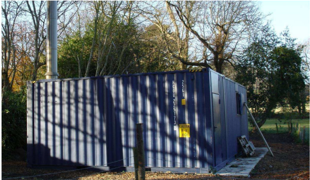
Figure 12 - Example installation - C/O Econergy
