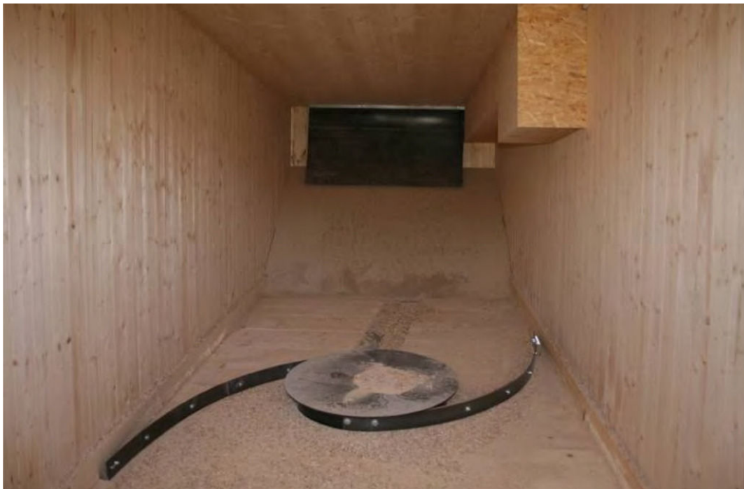
Figure 15 - Internal view of woodchip fuel storage container - C/O Econergy
