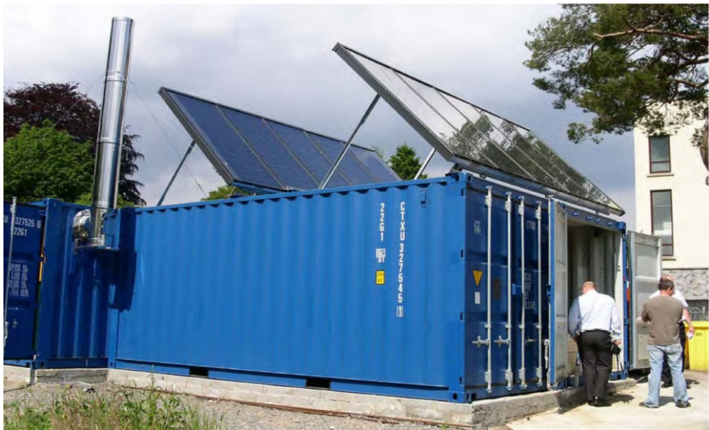
Figure 13 - Example installation - C/O Econergy
